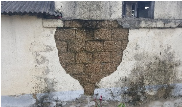
(c) Damage to concrete wall
