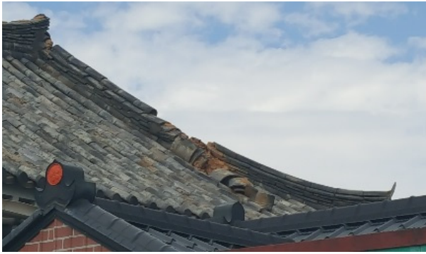
(a) Roof tiles falling off
