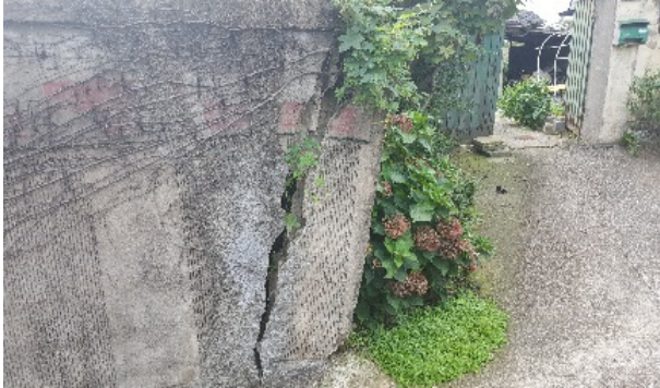
(b) Damage to concrete fence
