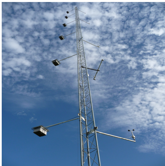
Figure 1. A 30 m tower installed with sensors at different heights to measure air temperature, wind speed, and wind direction.
