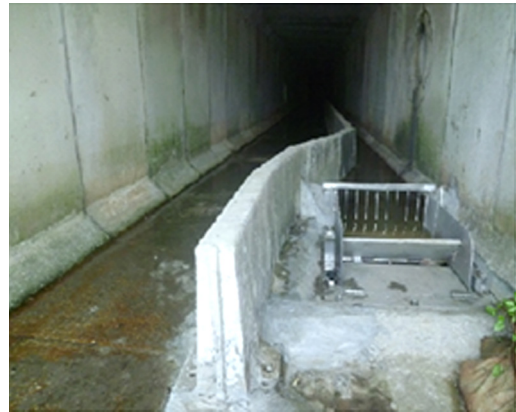
Fig. 3. Photo of inflow controller installed at the outfall.
