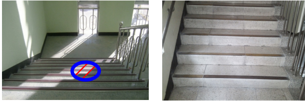
Figure 5. Accidents caused by non-slip (논슬립에 의한 사고)
