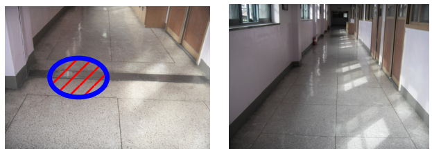
Figure 4. Lack of action on the connection part(연결부위 조치 미흡)
