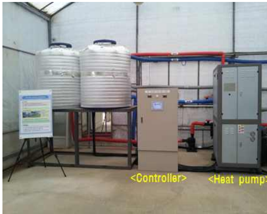
Fig. 2 System installation view
