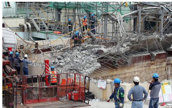
〈Fig. 1〉 Scene of explosion accident (2015. 7)
