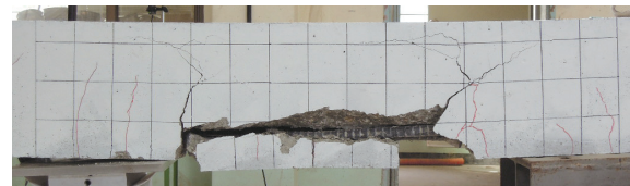
(b) Splitting failure of splice test
