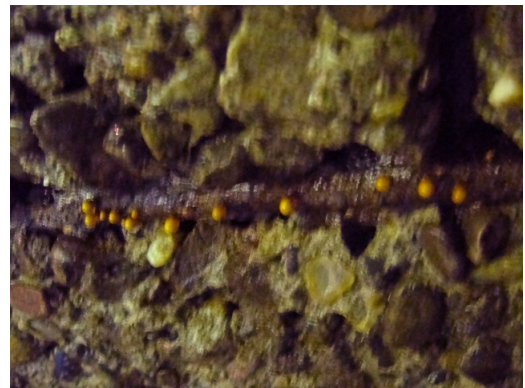
Fig. 6. Concrete interior exposure and reinforcing steel corrosion (elution)
