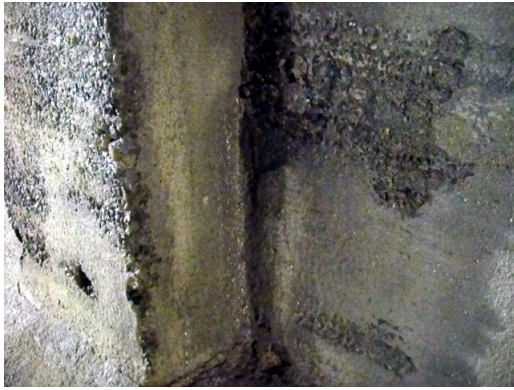
Fig. 7. Concrete weakening due to chloride and carbon (surface peeling by slight touch)
