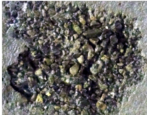
Fig. 8. Concrete aggregate exposure
