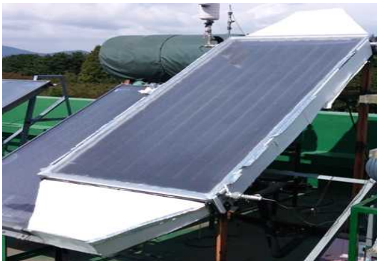
(a) Actual feature of hybrid solar air-water heater
