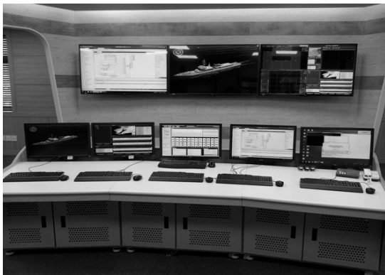
Fig. 15. QUEST Operation Control Equipment
