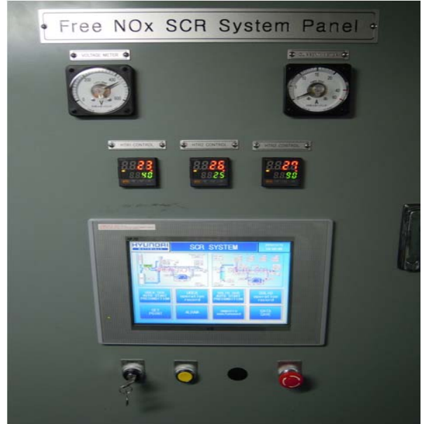
Figure 6: A PLC panel for the SCR system
