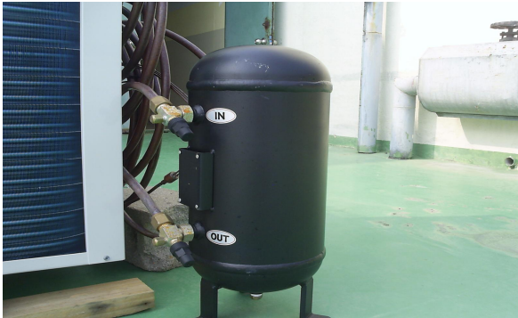
Fig. 3. Buffering Refrigerant Accumulator
