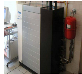
Fig. 8 Cogeneration system with Stirling engine/alternator(ENATEC)
