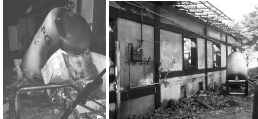
Fig. 1. Fire case caused by failed small-sized LPG storage tanks.
