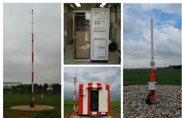
Fig. 2. Honeywell SLS-4000 installed at Gimpo airport
