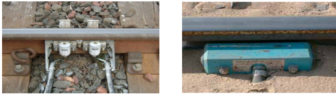
Fig. 3. Sensors installed on the rail
