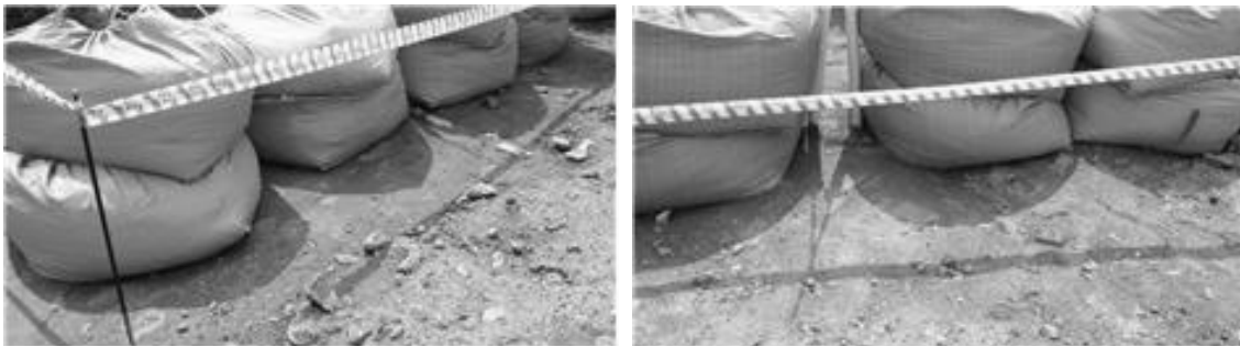
Fig. 14. Ground settlement in backfill material area
