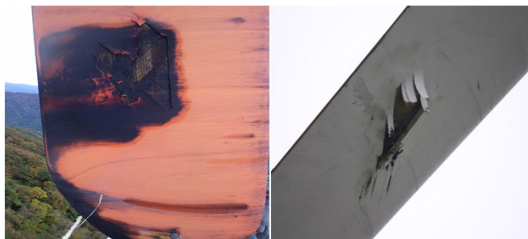
Fig. 10 Damage to blades by direct lightning (Left: TGS, Right: GW)
