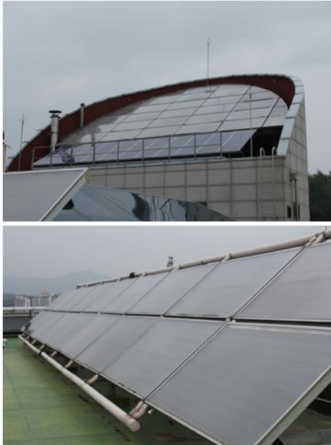
Fig. 2 Solar thermal collectors of the building
