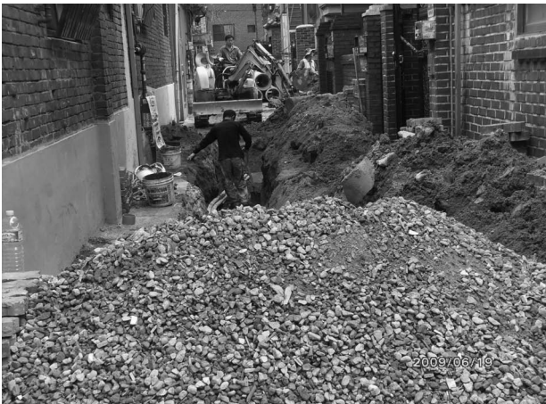
Fig. 2 Road Blocking due to Excavating Soil after open-cut Pipe Construction
