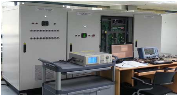
Fig. 8 30[kVA], 440[V] STATCOM system
