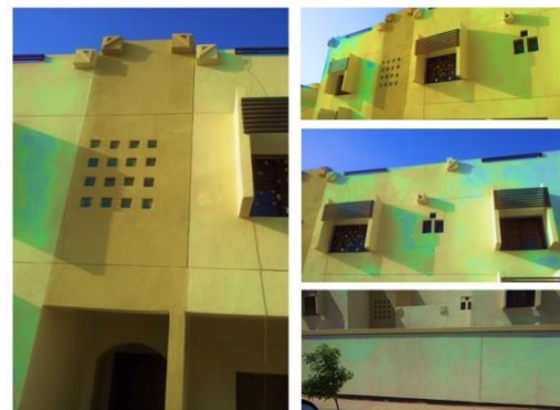
FIGURE I PHOTOS HIGHLIGHTING EXTERIOR QUALITY ISSUES
