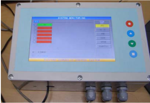
Figure 11: System Monitoring of Master Controller
