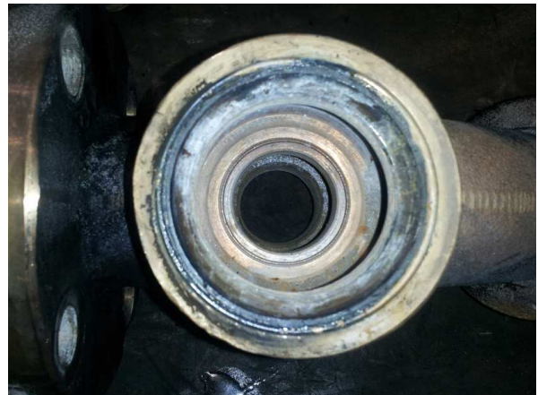
Fig. 3 Shape of valve seat after fire safety test
