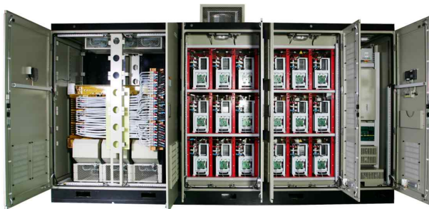
Fig. 11 H-bridge multi-level inverter hardware
