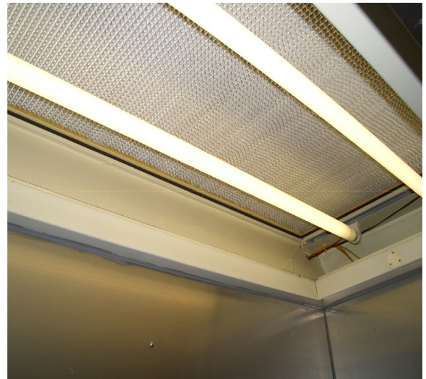
Fig. 1. Example of the faulty design of biosafety cabinets due to the fluorescent light, which was disturbing the tests for the downflow velocity and efficiency of the HEPA filters. HEPA, high efficiency particulate air.
