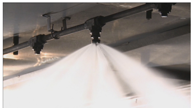
Fig. 4 Water-mist spray of nozzle C
