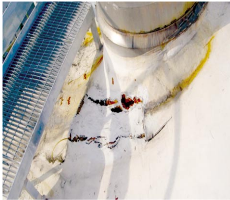
(c) Damage insulation
