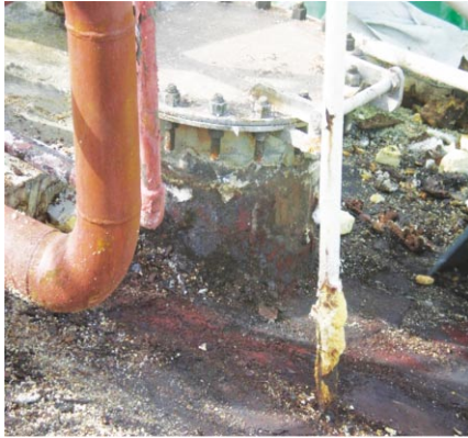
(a) Oxidation corrosion
