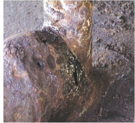
(b) Local corrosion
