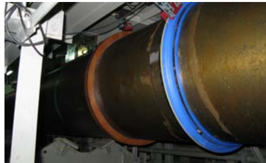
Figure 6: The EDiMS telemeter system installation with strain gage
