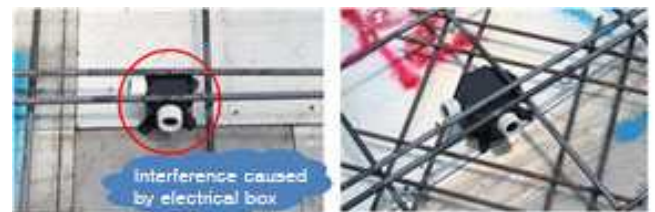
Figure 11. Failure of equipment and reinforcement in the slab
