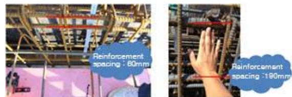
Figure 8. Rebar interval error
