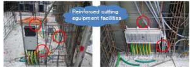
Figure 10. Wall of the horizontal and vertical rebar cutting error
