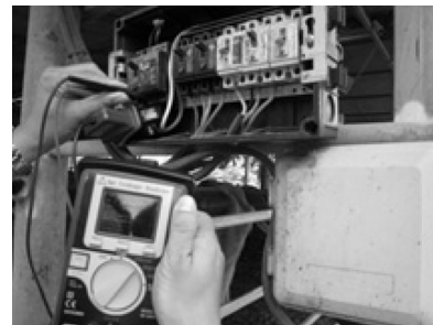
c) Measuring at panel
