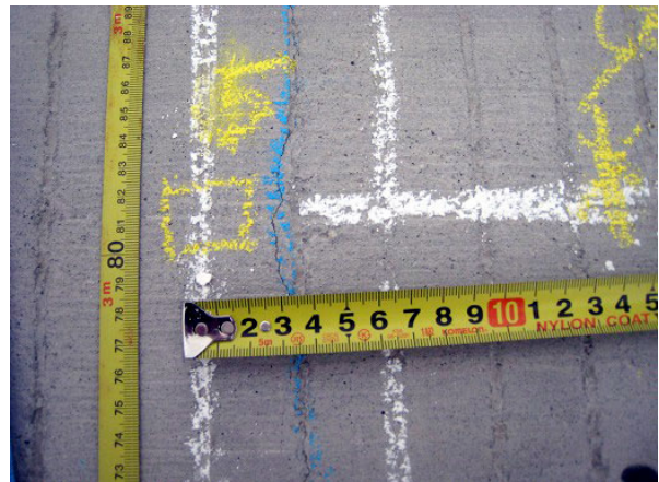
Fig. 10 Crack Occurrence at the Crack Induced Area
