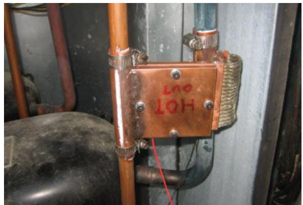
Fig. 1 The TEG Module Clamped to the Pipes of the Compressor
