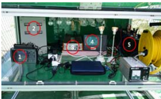
Figure 5: Internal appearance of hybrid power generation system
