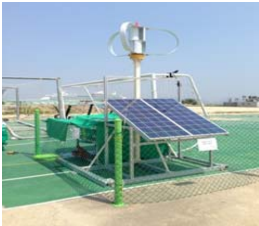
Figure 4: External appearance of hybrid power generation system
