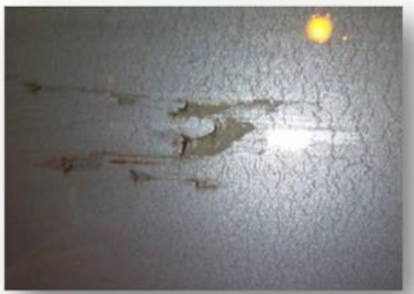
Fig. 1 H-beam web crack
