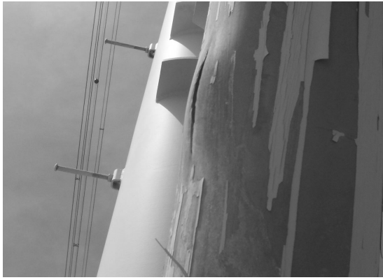
(a) Bulking damage for tower members
