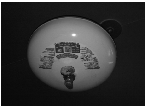
Figure 1. An automatic fire extinguisher.
