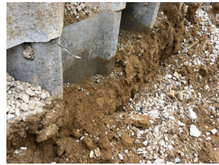
[Fig. 7] Omitted drainage layer from the back of block
