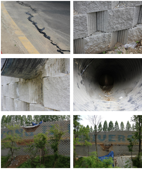
[Fig. 2] Cracked and collapsed reinforced retaining wall
