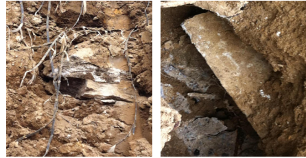
[Fig. 4] Boulder stone and waste concrete in back fill
