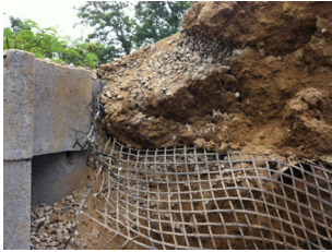
[Fig. 5] Damaged reinforcement by settlement
