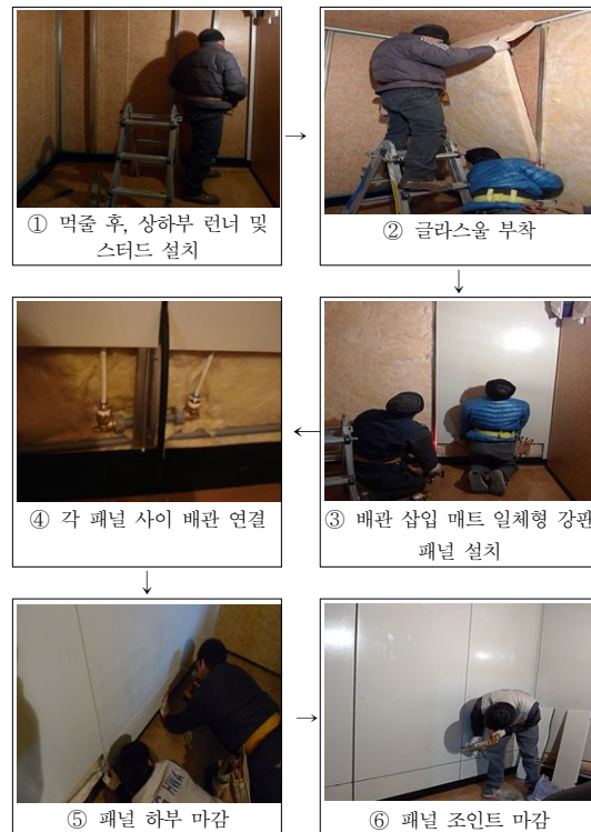
Fig. 5 Installation processes of prefabricated steel wall panel for radiant heating and cooling
