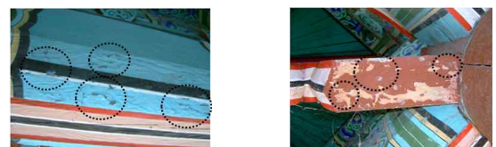
a) Dancheong Exfoliation b) Efflorescence and Dancheong Drop Out Figure 2. Efflorescence phenomenon on the Dancheong
