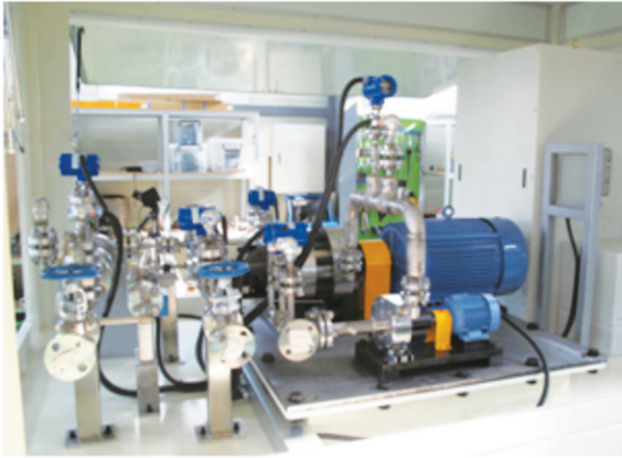
Fig. 3 Pilot-scale CO 2 injection system
