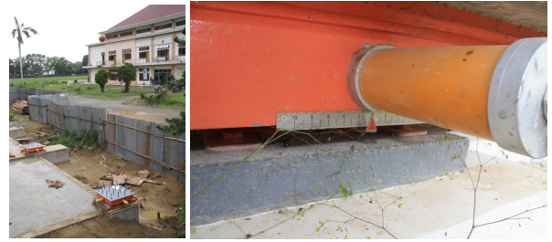
Fig. 17. Installation of EQS and picture of EQS after earthquake
