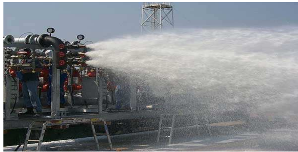
Fig. 1 Water deluge system on working
