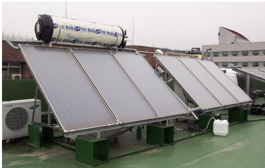
Fig. 1 A photo of a passive and an active type solar water heating systems
