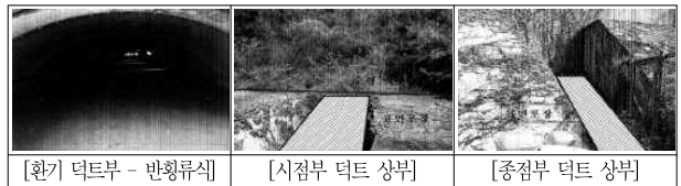
〈Figure 6〉 Ventilation of Namsan No.2 tunnel
