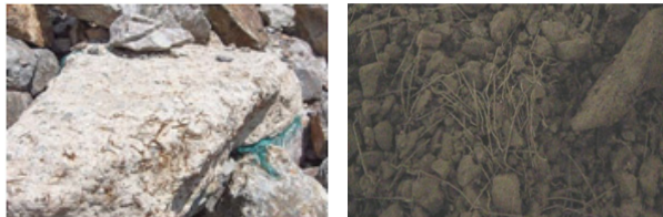
(b) Corrosion of steel fiber
