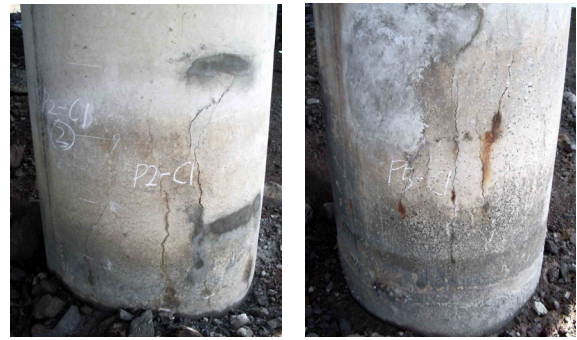
Fig. 4. Results of view inspection (Left: P2C1, Right: P5C1).
