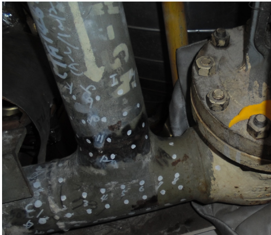
Fig. 3. Picture for thickness measurement.
