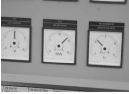
Power meter (14 MW)
