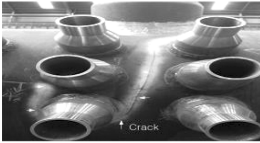
Fig. 7 Main crack on base metal & HAZ
