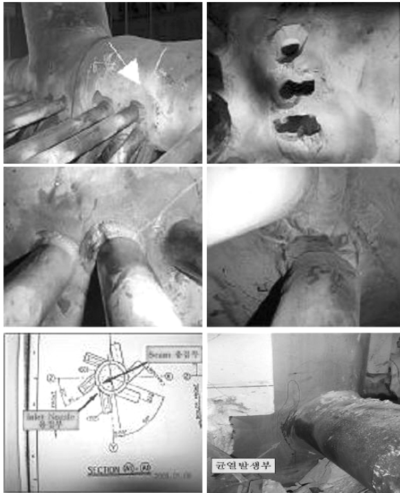
Fig. 10 Example failures on narrow weld-joint and cross weld metal 4)
